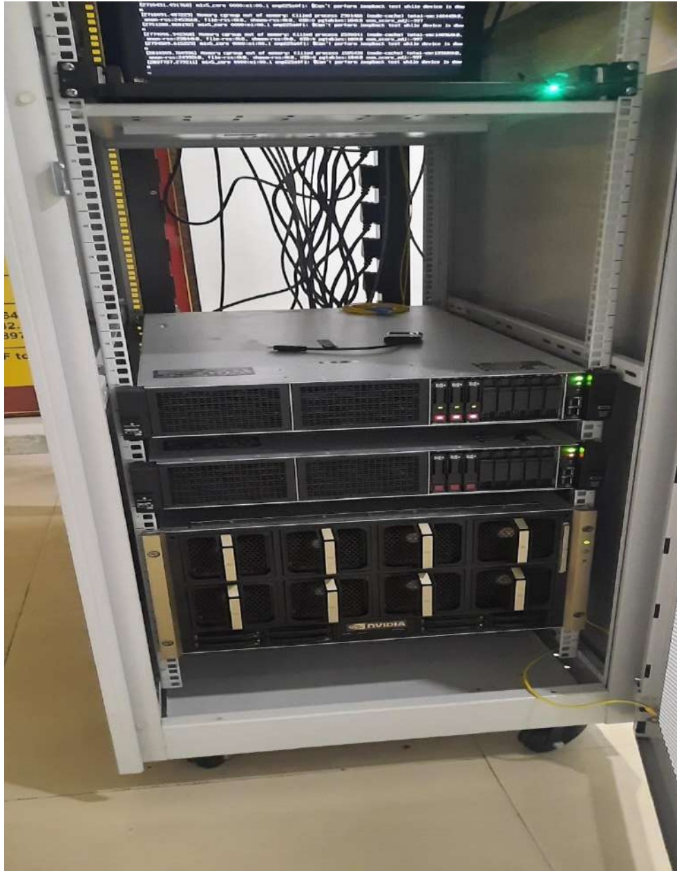
Figure: Server Room
