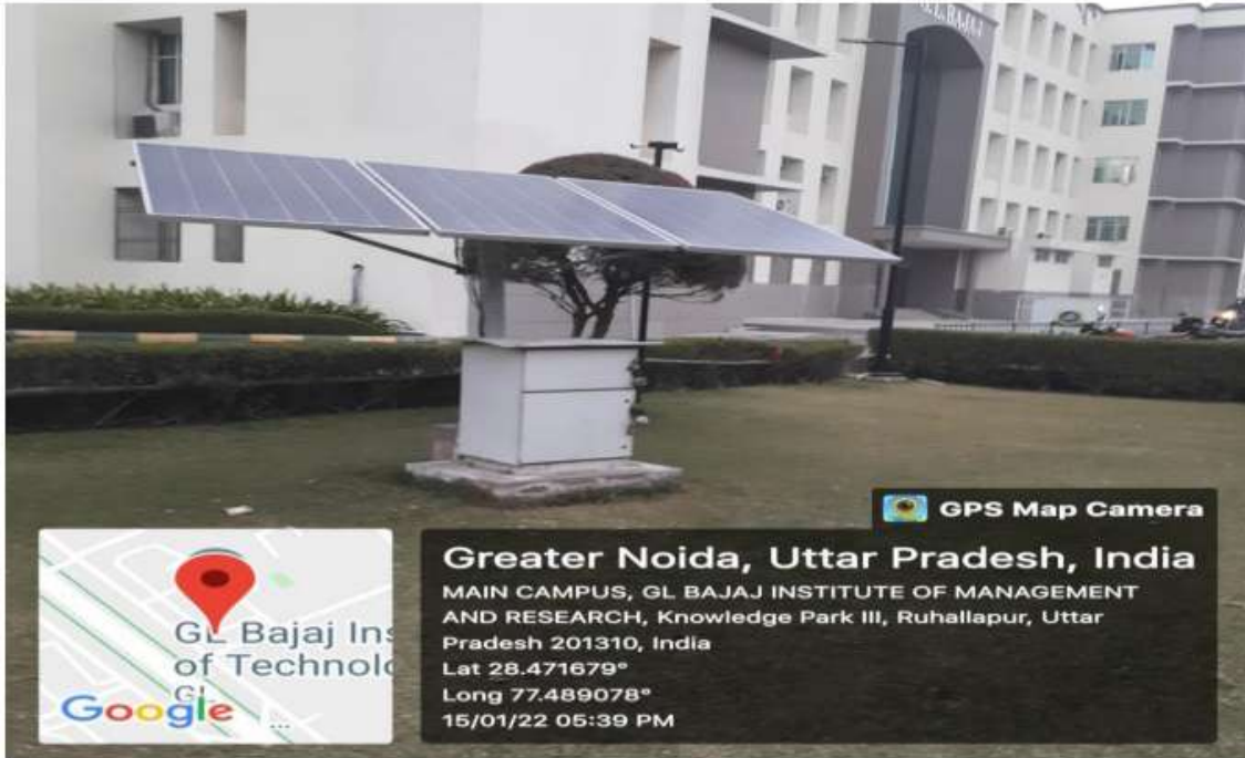
Solar energy based electric vehicle charging Unit
