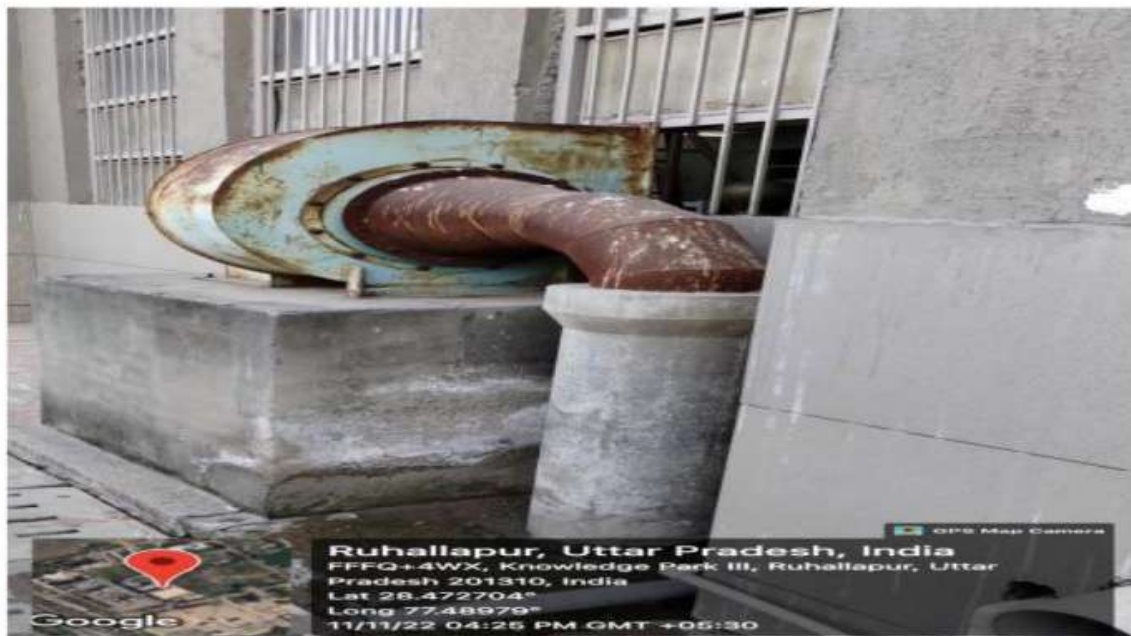
Geo-thermal based temperature control system
